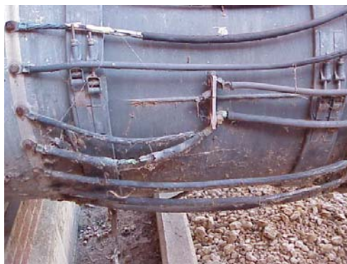
FIGURE 8: In some cases a visual inspection will located deteriorated external jumpers.
