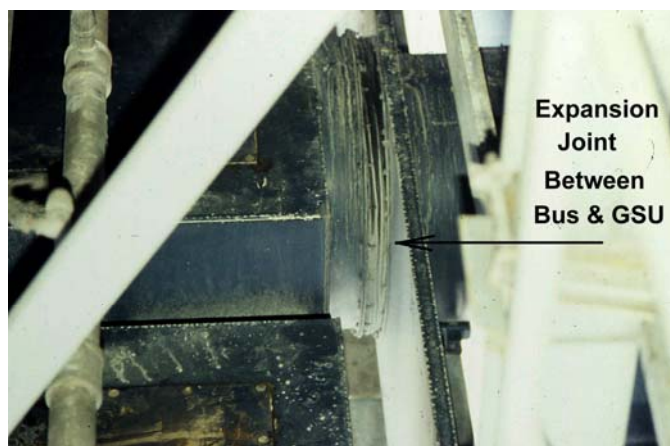
FIGURE 21: Deterioration of the air seal between bus and GSU can be expected.
