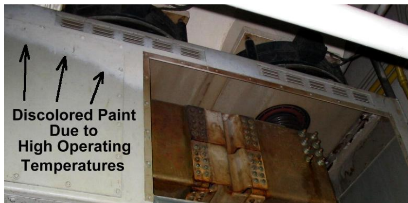
FIGURE 22: The neutral enclosure under a generator is a section of bus often over looked.
