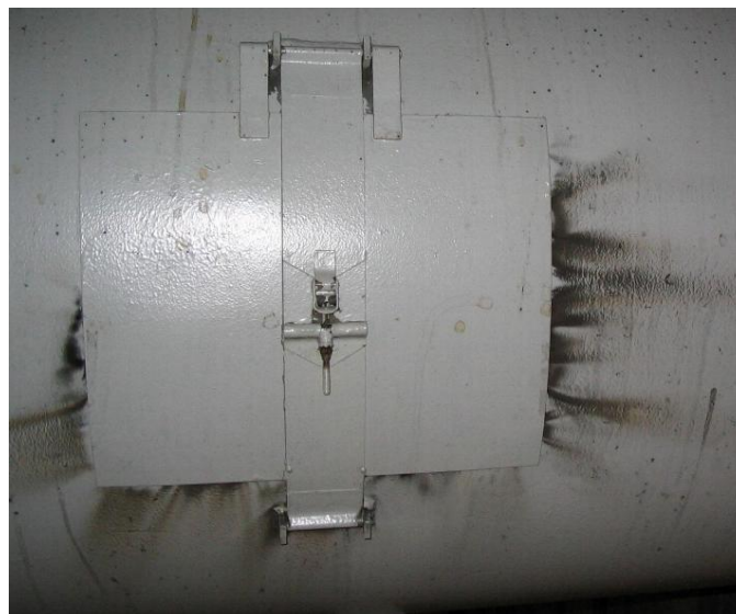
FIGURE 20: Forced air-cooled isolated phase buses often develop air leaks around the inspection hatches due to hardening of the original gasket material.
