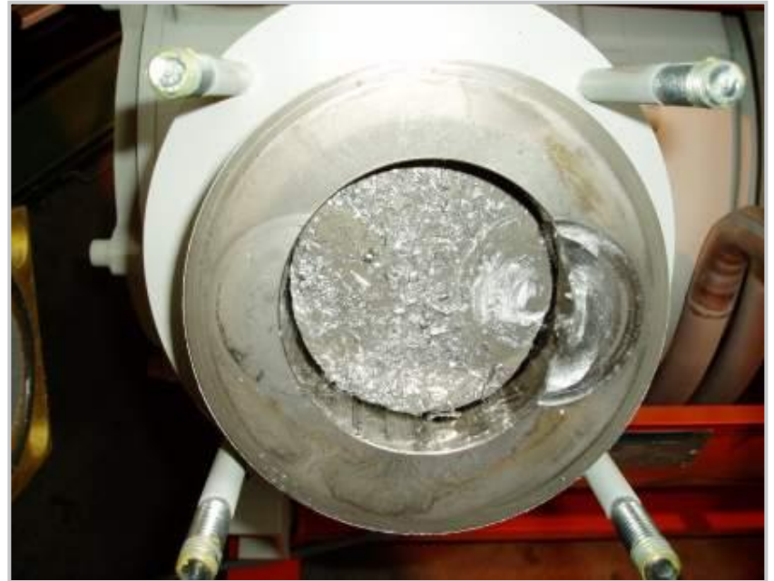
Inadequate maintenance of gas handling equipment
