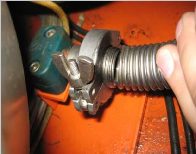
Gas leaks on pipework system
