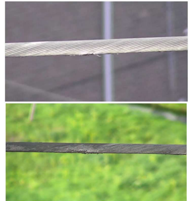
Conductor Broken Strands
