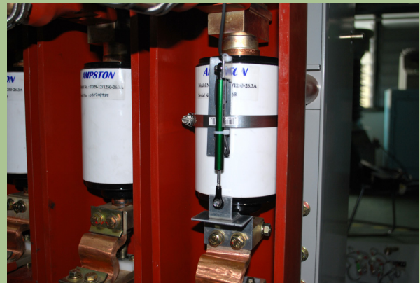
Resistor Transducer on a Vacuum Circuit Breaker
